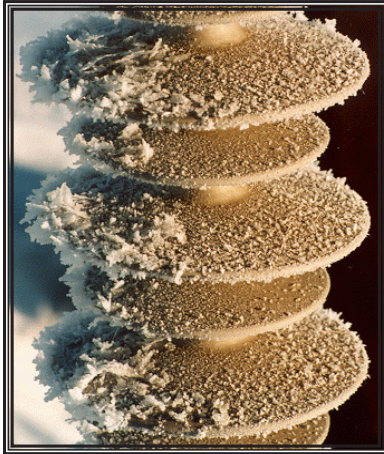
Condensation on Switchgear Insulators
