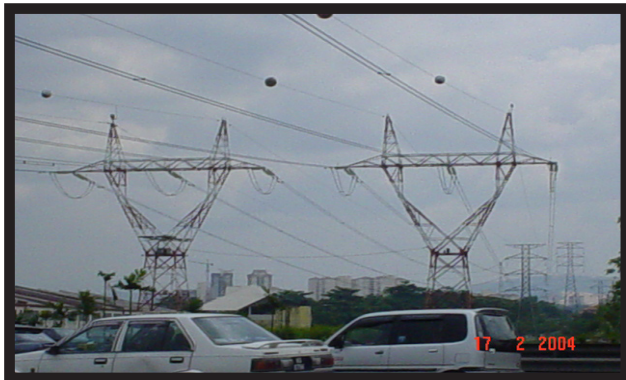
TNB Overhead Line
