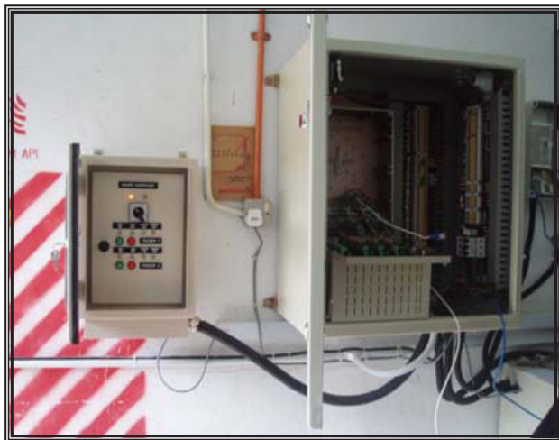
RTU and Control Panel
