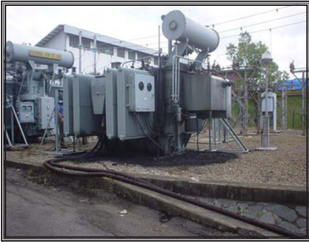
Distribution Transformer used in the project to assess its Risk Index
