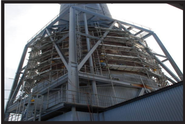
Putrajaya Power Station's Exhaust Gas
