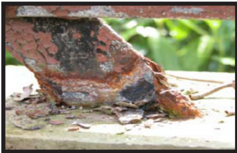
Typical corrosion at tower foot caused by wet-dry condition in
