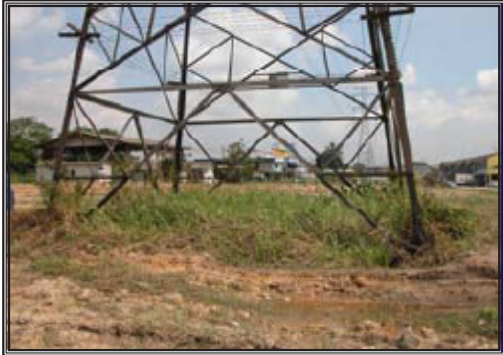
Condition of soil at ground level of tower that contributes to high level of
