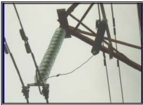
SEDIVER TLA (SLA) installed on Balakong to Serdang 132kV line
