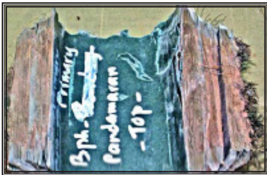
View of damaged VT
