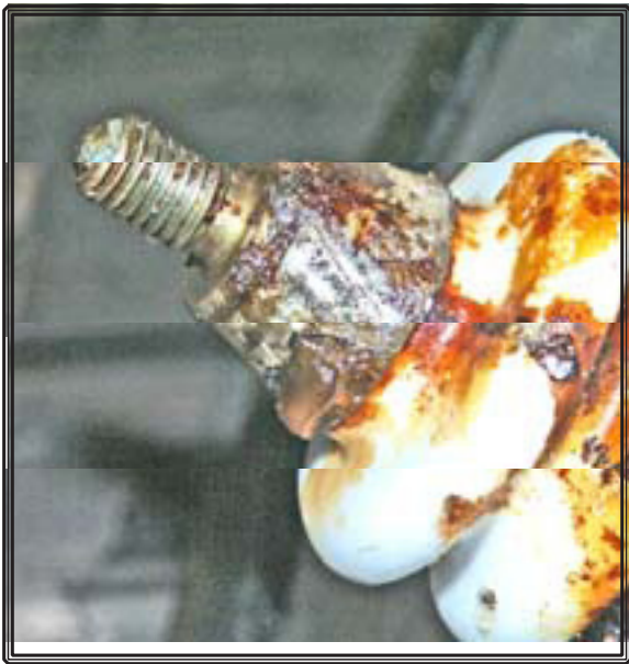
Heavy sludge contamination on the insulator surface
